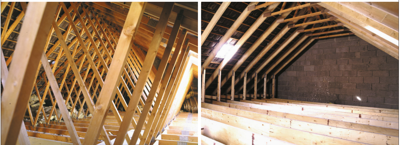
Figure 2.55. Conversion of nail plate truss structure to room-in-roof attic. Top and bottom cords have been reinforced with LVL-P beams and truss diagonals removed. LVL-C or plywood is used for the frame corner connections.
