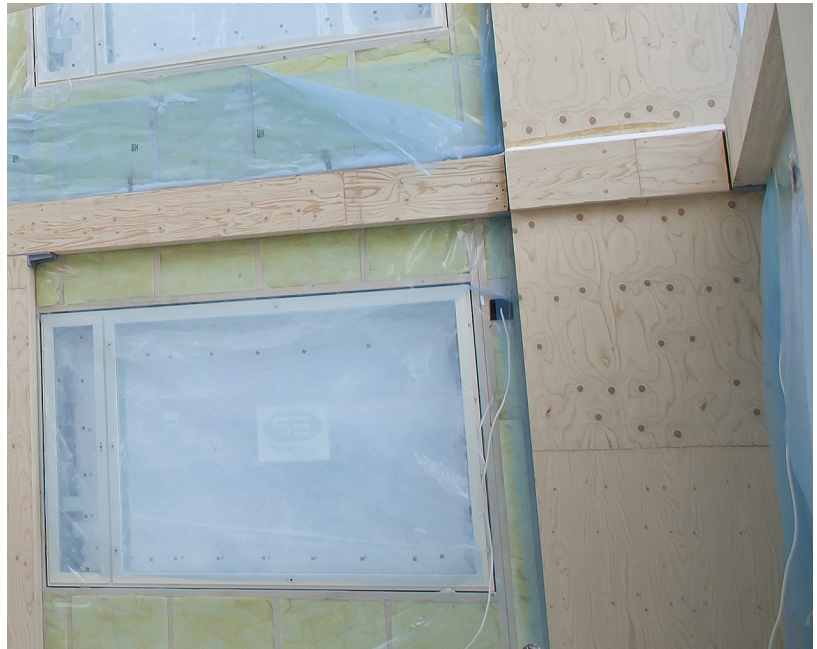
Figure 2.72. LVL-C bracing panels.
